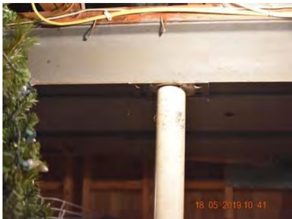
05/22/2019 Pictures of the support system.
